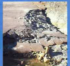
Washed out concrete at tunnel (BEFORE)
